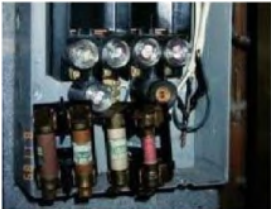
FUSE BOX FUSES
