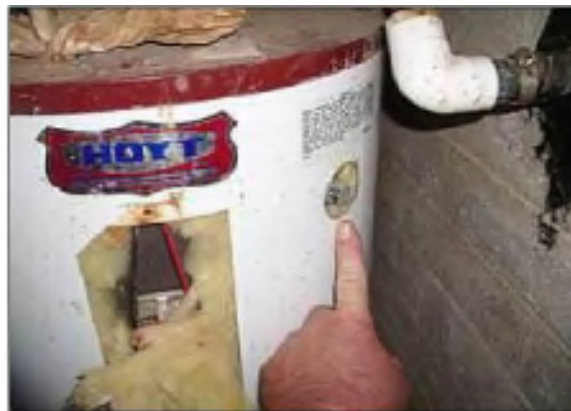
MISSING TPR VALVE
