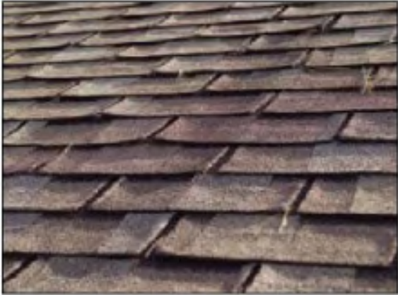
LIFTING/ CURLING SHINGLES
