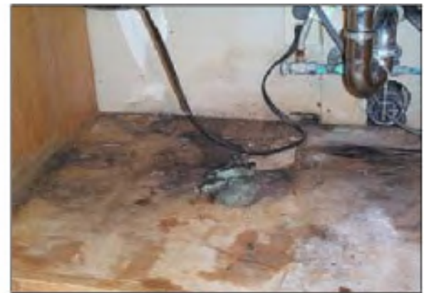
EXISTING WATER DAMAGE
