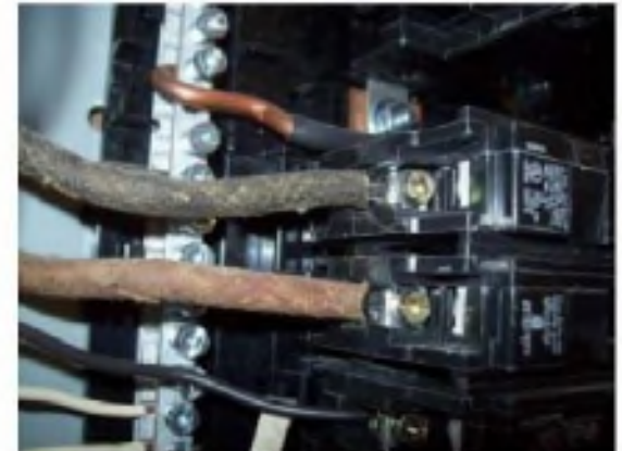
CLOTH SHEATHED WIRING
